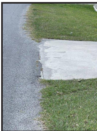
Not good for water runoff
